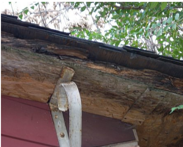
Wood rot on garage
