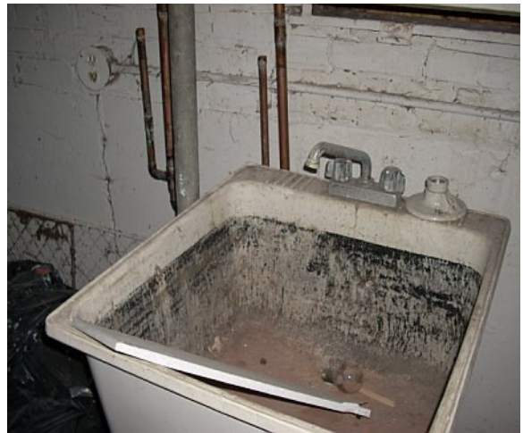
Mold in basement tub
